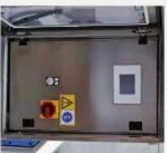
Control panel of industrial dust control system Giraffa
