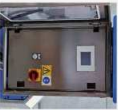
Control panel of industrial dust control system Elefante
